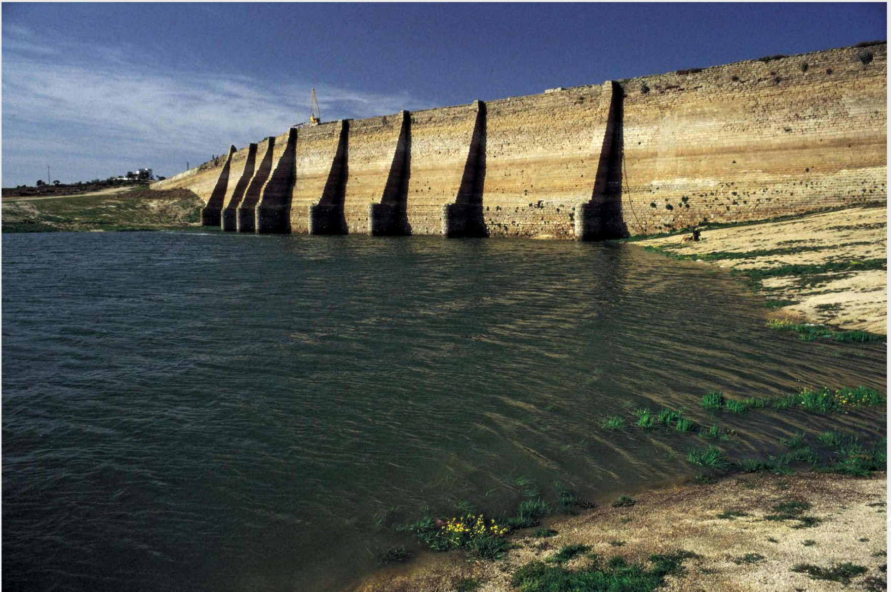
Proserpina Dam, Spain emptied reservoir from the upstream side Height: 12 m, Length: 428 m
